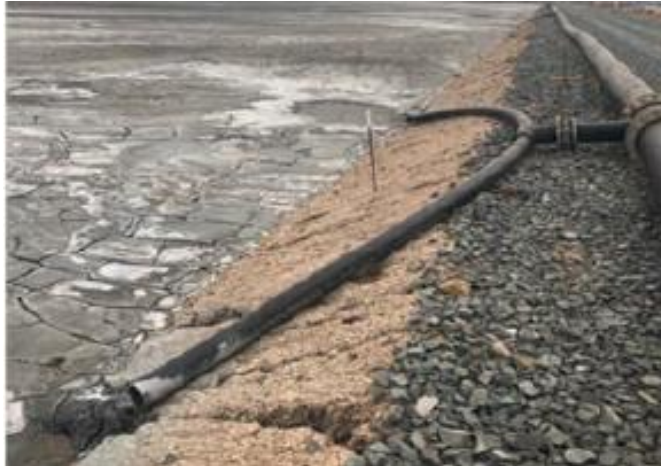
Droppers near the discharge point on eastern wall, Stage 5
