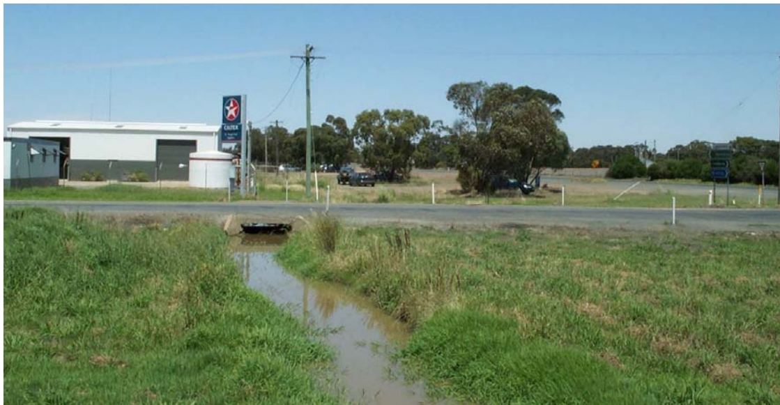
Photograph 8 Erosion at Showground Road
