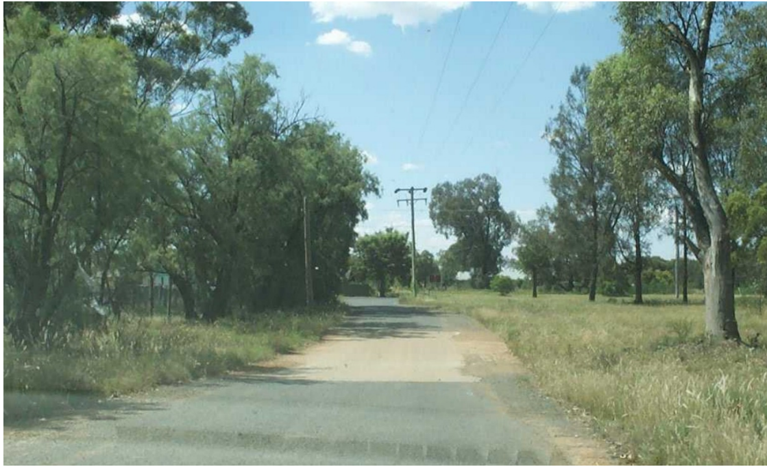
Photograph 9 Sedimentation at Sewage Works entrance
